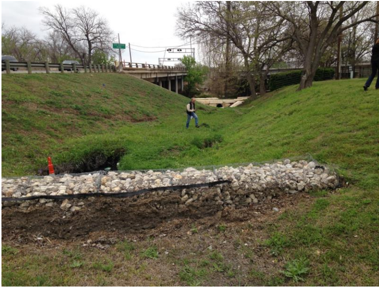
Figure 8-25 Photo of Storm Sewer Outfall below Grade and Poned Water
